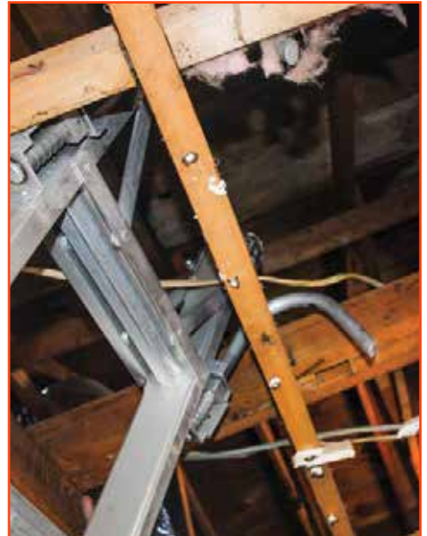
Roof / Rafter hooks
